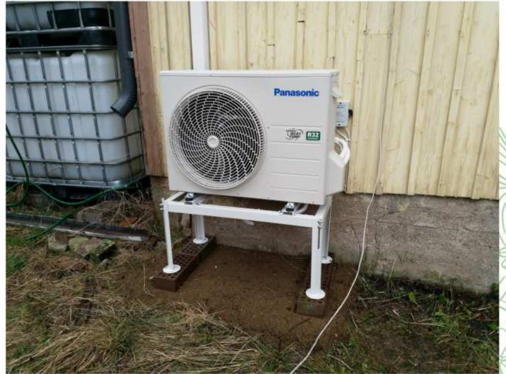
Image 13: installed electric heat pump, external unit, May 2023
